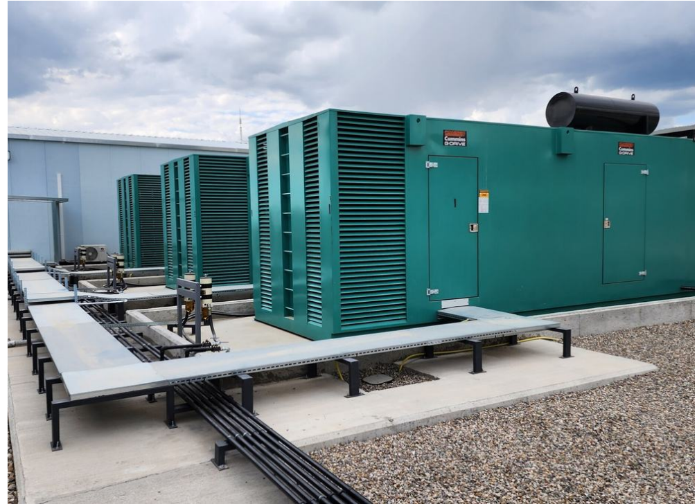
■ Containerized generator plant with cable trays, military base installation
