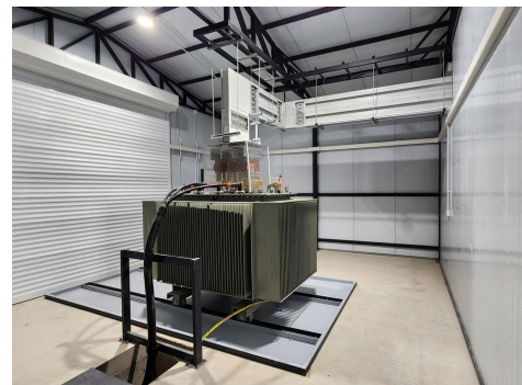
■ Transformer room and switchgear
