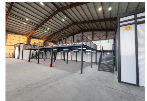
■ Steel mezzanine offices inside a warehouse
